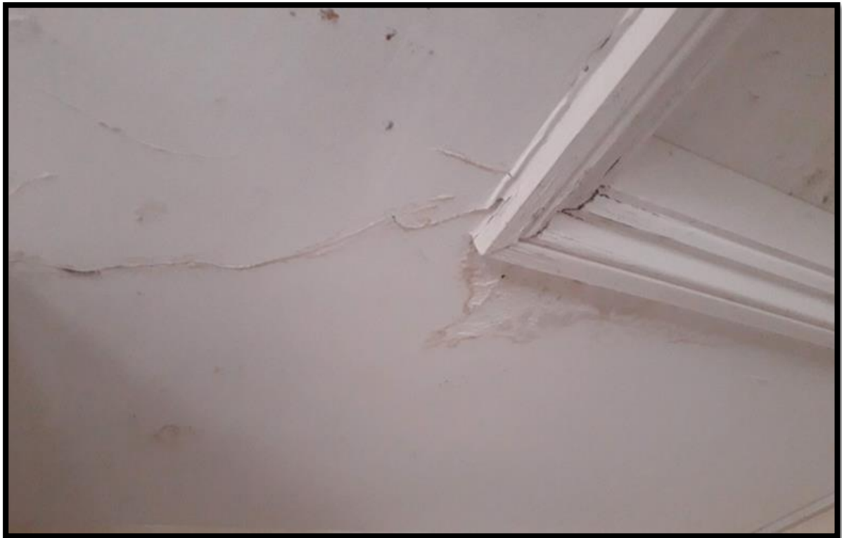
Water damage to ceiling due to water ingress prior to roof repairs.
