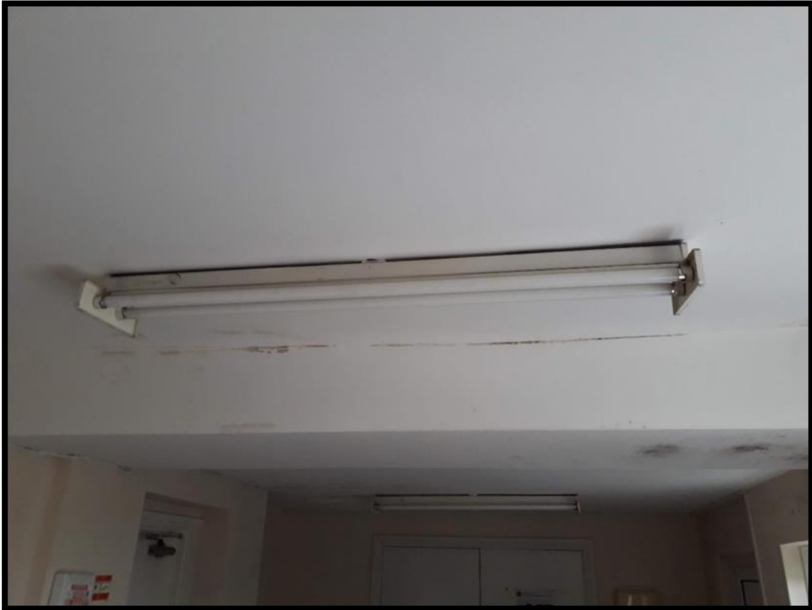
Current strip lighting.
